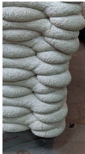
Figure 14. Vertical cracks along the ribs
