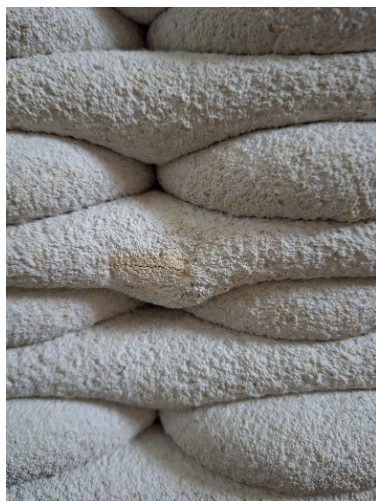
Figure 13. Horizontal crack with pigmentation
